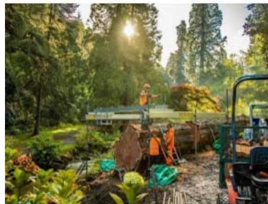
Contractors working on the fallen Sequoia sempervirens .
